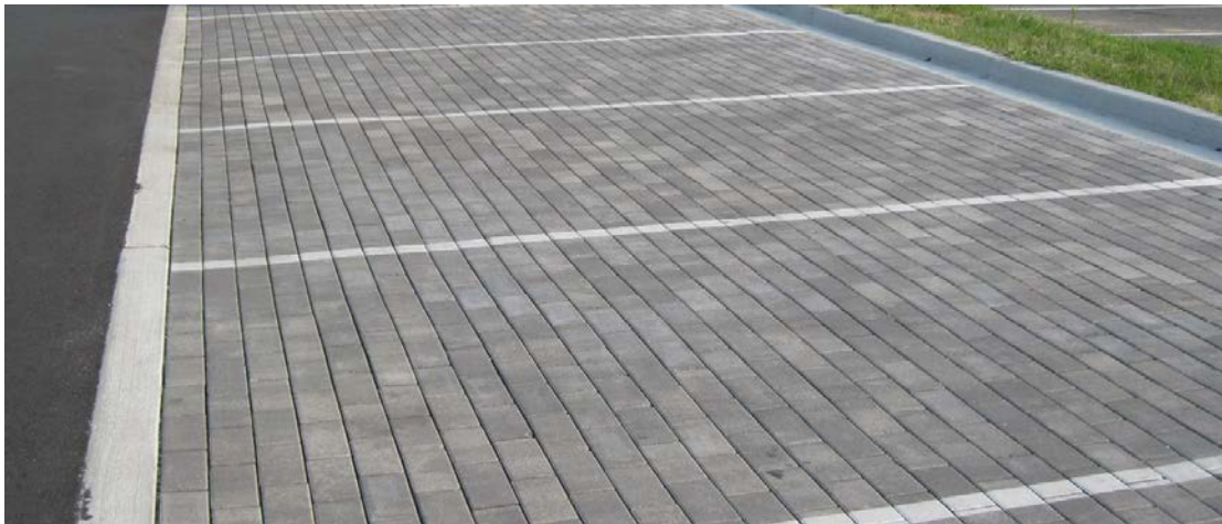
Figure 1 Permeable Concrete Pavers (Source: Fort George G. Meade Department of Public Works)
