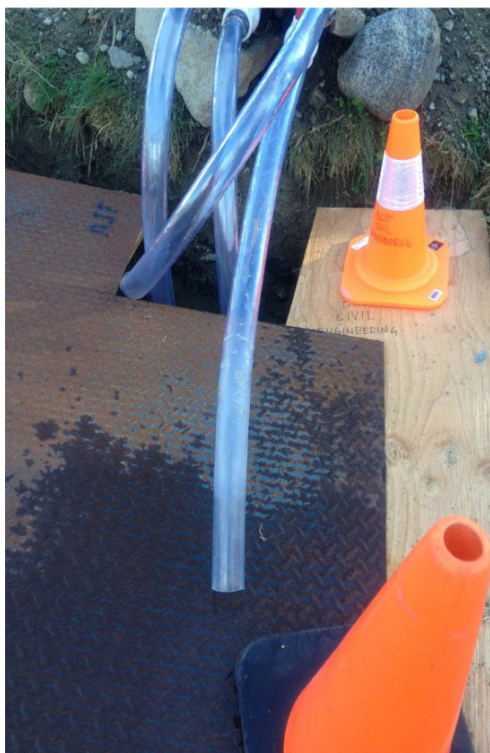
Photo 3. Downstream end of pipes feeding into a collection chamber.
