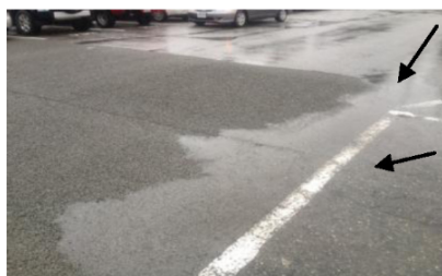
Photo 12. Run-off being captured by pervious concrete.
