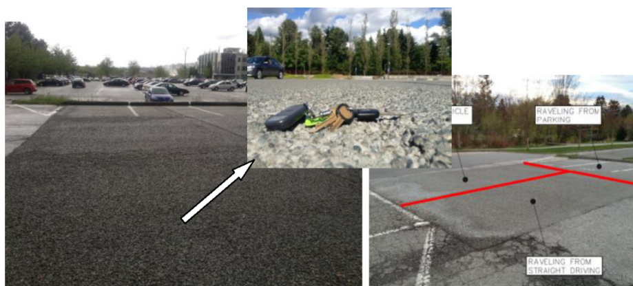
Photo 10. Current state of raveling in pervious concrete after 40 weeks in service.
